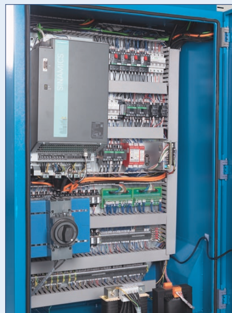
A heat exchanger ensures reliable operation of control electronics under continuous operation
