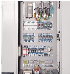
The large control cabinet is equipped with high-quality components
